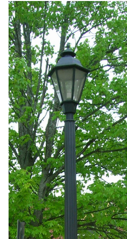
Figure 4-3: Pedestrian light components: Luminaire and pole
