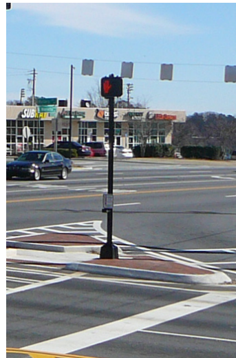
Figure 8-2: Pedestrian signal pole
