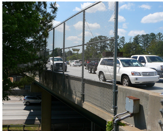
Figure 11-3: Existing chain link fence on bridge at Holcomb Bridge Road and GA 400.
